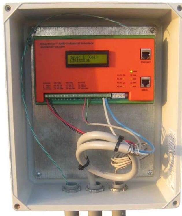
An Installed EtherMeter™ AMR-Industrial Interface
