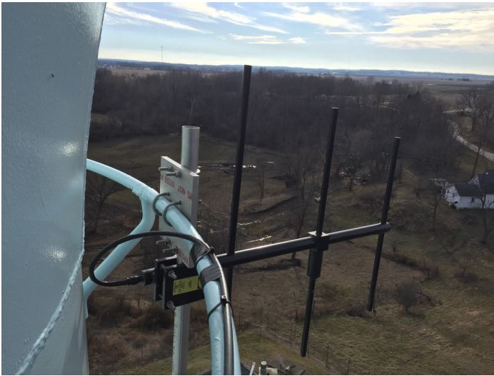
Rear View: VHF Yagi SCADA Antenna Mounted To Painter Rings Using the PTM-90 Mounting Kit
