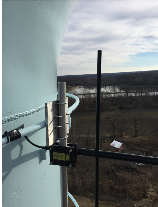
Front View: VHF Yagi SCADA Antenna Mounted To Painter Rings Using the PTM-90 Mounting Kit
